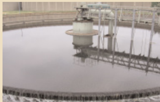
Activated sludge is settled out in this clarifier. Flow enters the tank from the top and flows radially outward.
