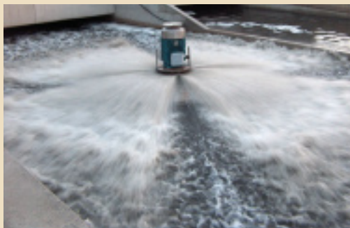
The surface aerator of this bio-reactor is used to resuspend the solids bed from within an aeration lane and to entrain air into the reactor.
