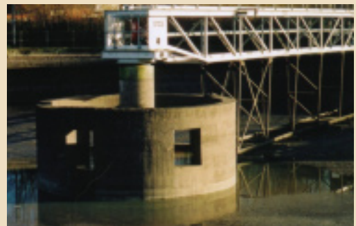
Storm settling tank influent
